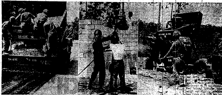
GRAVEL POURED ON MOYE RD., SPOTLIGHTS INSTALLED AT BLOCKHOUSE, FOUNDATION PREPARED BY GEAR-LOADED ENGINEERS. Projects were Part of the 43rd Engineers' Three-Day Army Training Test Last Week (Photos by S. Sgt. Betty Farmer)
