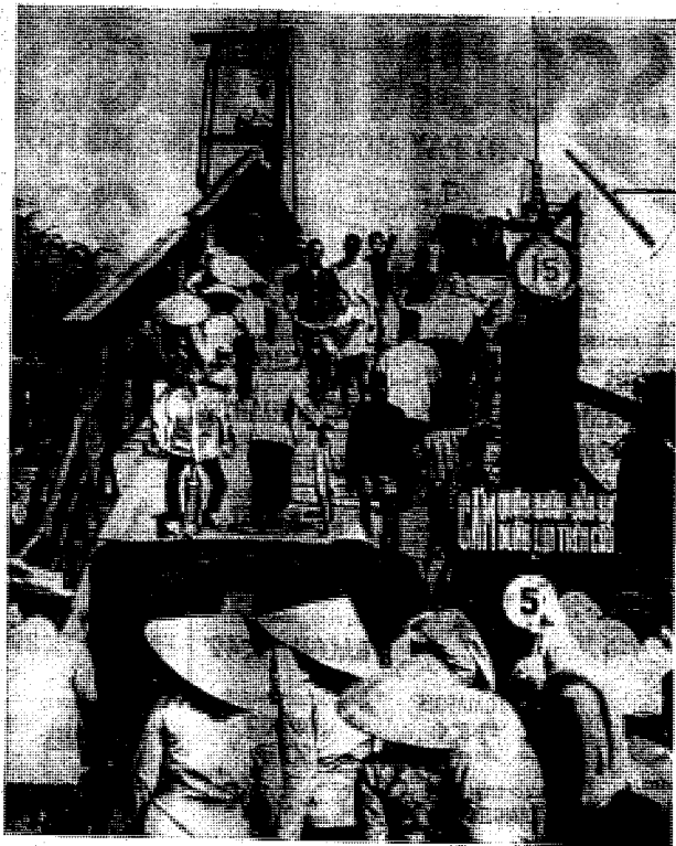
MADAM NHU'S BRIDGE . . . BAC LIEU CANAL BRIDGE WAS REBUILT AT STEEPER ANGLE Old Bridge Would Not Accommodate Mast of Madam Nhu's Pleasure Craft
